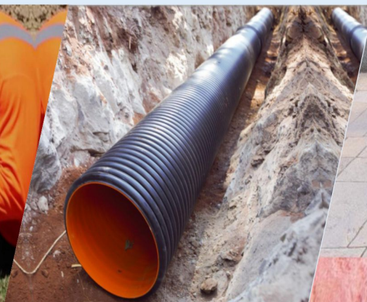
Underground Sewer Pipe Line
